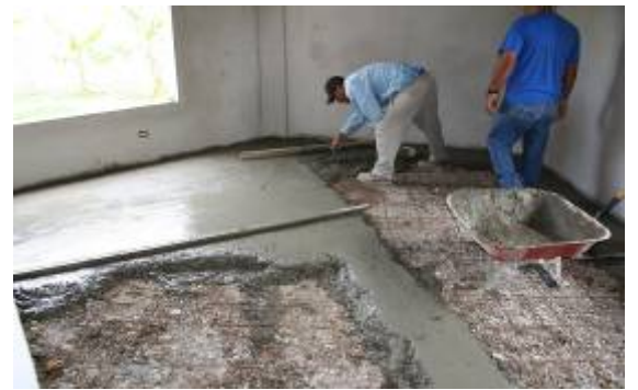
Site contractor, Mauricio, and Pastor Luis pouring concrete on the first floor
